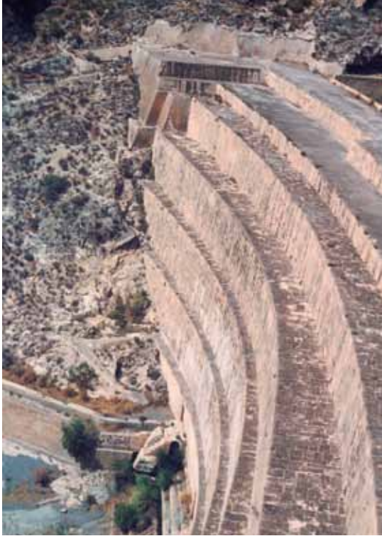
Figure 3. The Nijar reservoir (downstream view): a 35 m high hydraulic work built in the 1850's using ashlar. Image J. Porta.
