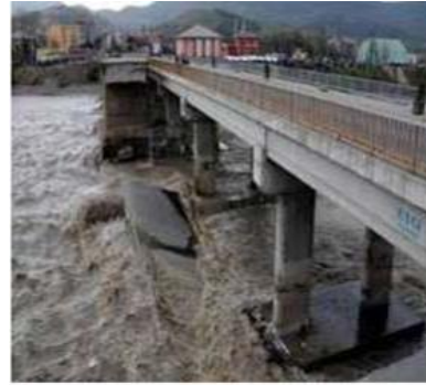
Picture 7. A collapsed bridge flood
