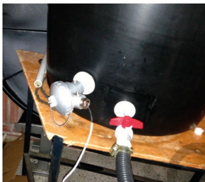
Fig. 2. Installed temperature sensor. Source: Authors
