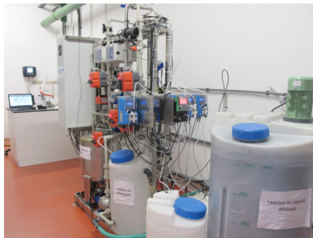
Figure 2. PAC/MF prototype designed by LNEC and installed in Alcantarilha WTP (LIFE Hymemb).
