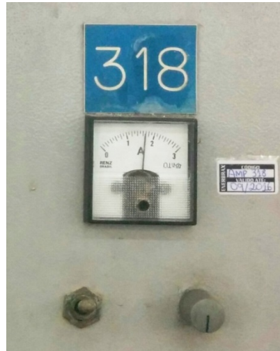
Figure 2: Manual power supply control devices.
