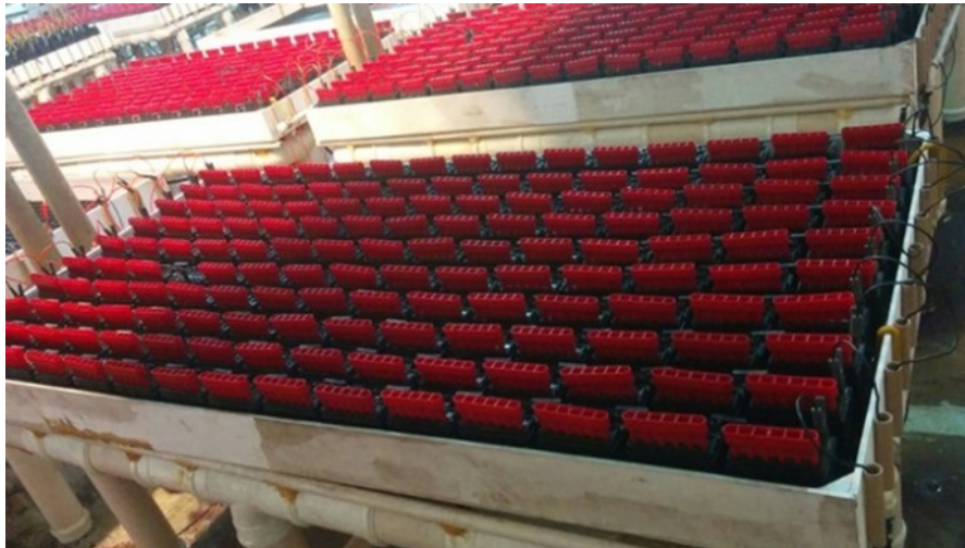
Figure 3: Batteries positioned and ready to connect the source of electric current.
