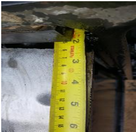
Fig 3. Fissure Length since pin separator to frame.
