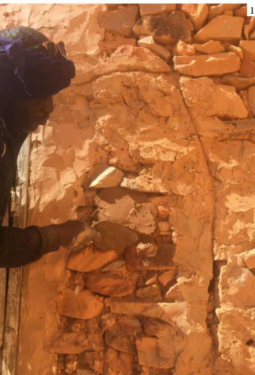
1: Local craftsman working on the finishing of an exterior wall 2: Tests of several mixtures for the finishings (Carmen Moreno)
