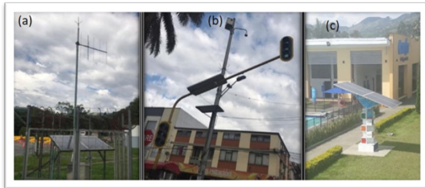
Figure 5. a. PVSS municipality of Chinchiná, La Pesebrera. b. PVSS camera and traffic light municipality of Chinchiná. c. PVSS charger of mobile equipment La Rochela.
