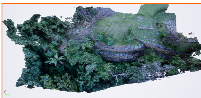
Figure 10. Photogrammetric recreation of the west retaining wall. Photos by A. Burbano, processed by Z. Meyer, 2020.
