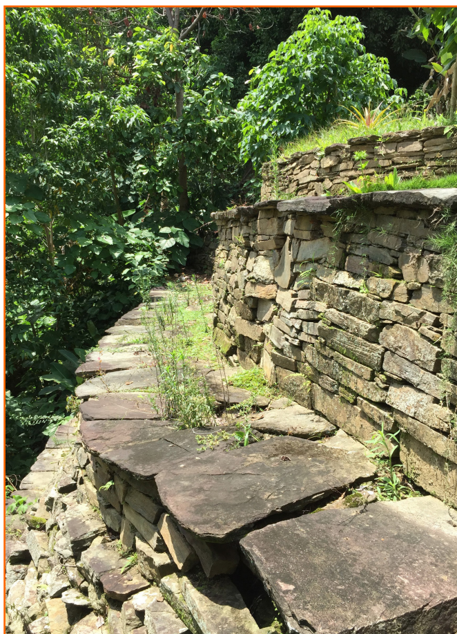
Figure 4c. Retaining wall on the west side of main terraces in CA. Photo by E. Mazuera
