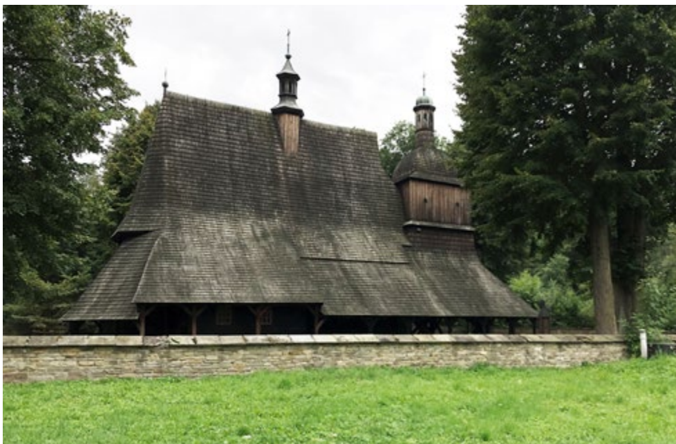
Monumental roof of the Church of St. Philip and St. James in Sękowa, Poland
