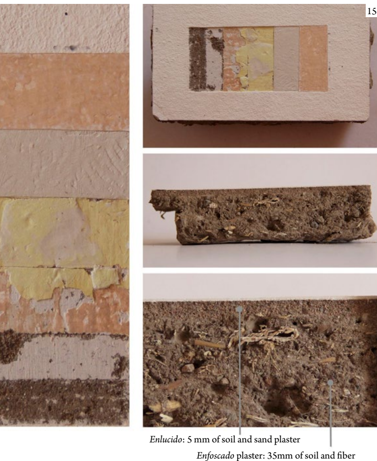
Figure 15: Indoor finish from the Corazón de María Convent in Ovalle (OVA02A). Left and top right: stratigraphic survey showing different layers of lime finishings and vinyl paints. Right center and bottom: section showing 5 mm of an earth and sand plaster ( enlucido ) and 35 mm of enfoscado with earth and fiber.
