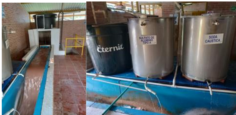
Figure 2. a) Rapid mixing (Parshall flume) b) Tanks with Coagulant and pH Corrector
