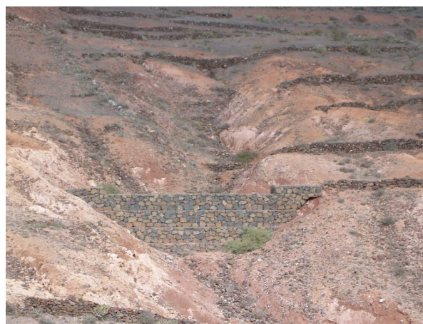
Figure 5. Gabion drop structure to reduce erosion
