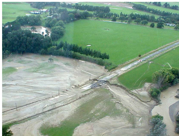
Figure 2. Road blocked by floods (Source: Civil Defence, New Zealand [2007])
