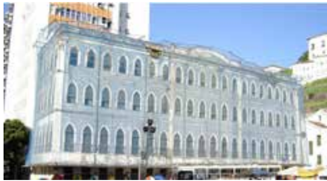
Fig. 15. Neo-gothic building protected with safety nets in Cairu Square, Salvador, capital of the state of Bahia. [Nivaldo Andrade]
