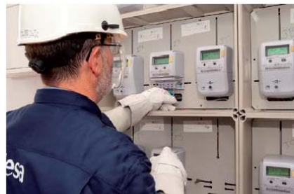
Figure 2. Placement of smart meters by an Endesa operator in the Smartcity in the framework of Málaga Project. Source: [3]
