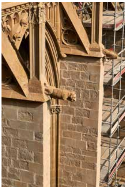
Contrafuertes, gárgolas y pináculos del ala norte del claustro de la Catedral de Pamplona Buttresses, gargoyles and pinnacles for the northern aisle of the cloister of Pamplona Cathedral
