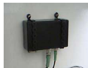
Figure 3: Photograph showing ADEX CM in plant
