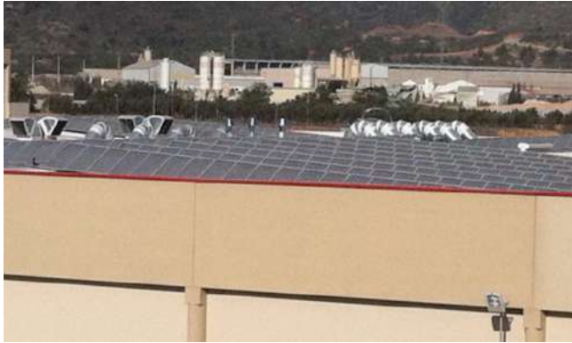
Figure 8. Detail of photovoltaic systems installed on the ground and on the roof. Source: own elaboration.
