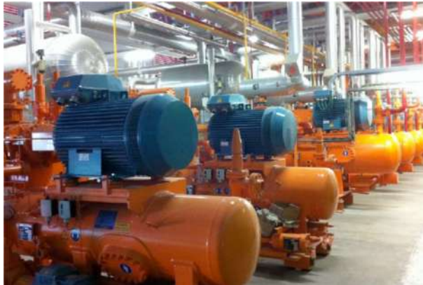
Figure 7. Detail of the technical industrial refrigeration room, designed for optimal energy efficiency conditions.
