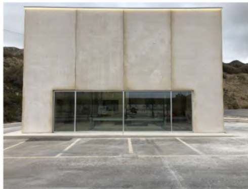
Figure 15. Appearance of the geopolymer façade on September 1, 2021, 138 days after its manufacture.
