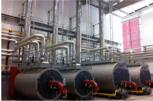
Figure 3. Detail of the boiler thermal technical room, designed for the correct maintenance functions.
