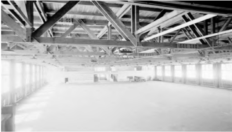
Figure 5. Wooden beams of the former University of British Columbia Armoury Source: Ross, (2020).
