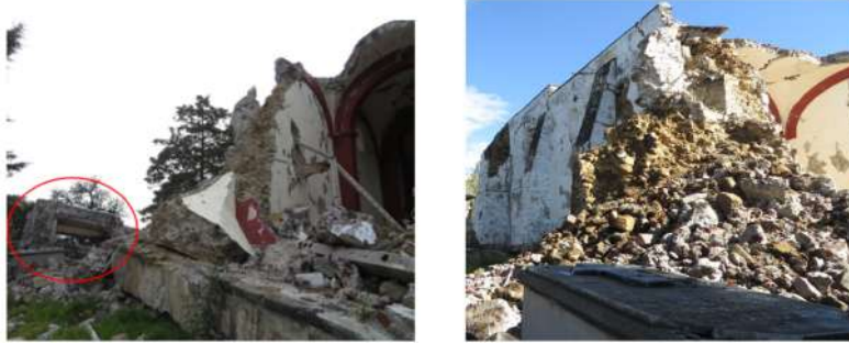
Figure 7. typical seismic damage in earthen constructions by the 2017 Puebla-Morelos EQ, Mw= 7.1 and 8.2,
