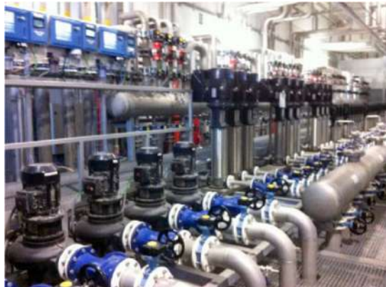
Figure 6. Detail of fluid rooms, with regulation systems using electronic drives.
