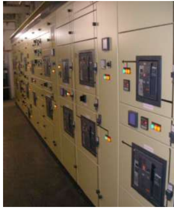
Figure 5. Detail of control and monitoring systems in general tables.
