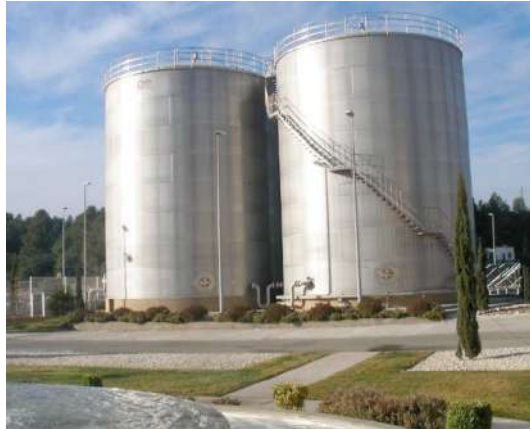
Figure 10. Detail of rainwater storage tanks.
