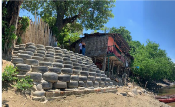
Figure 10. Wall in tyres in the fishermen's port ( 2020)
