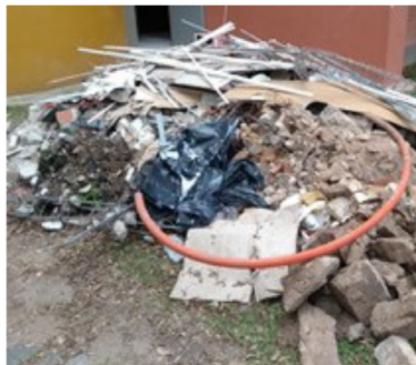
Figure 2. Different construction materials from demolitions and collapses.
