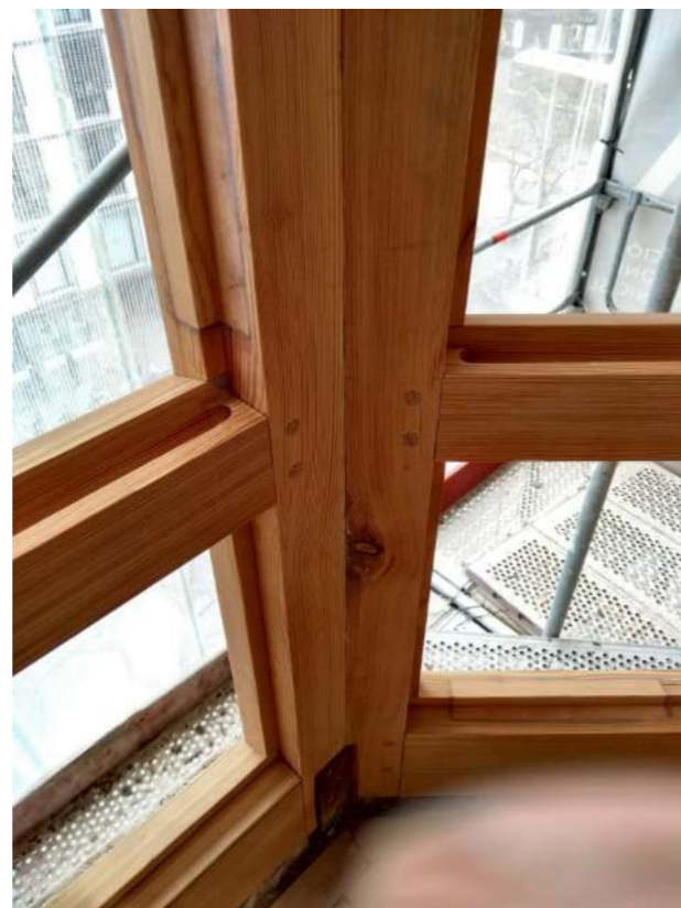
Restoration of a wooden bay window structure on an Art Nouveau building in the Eixample district of Barcelona
