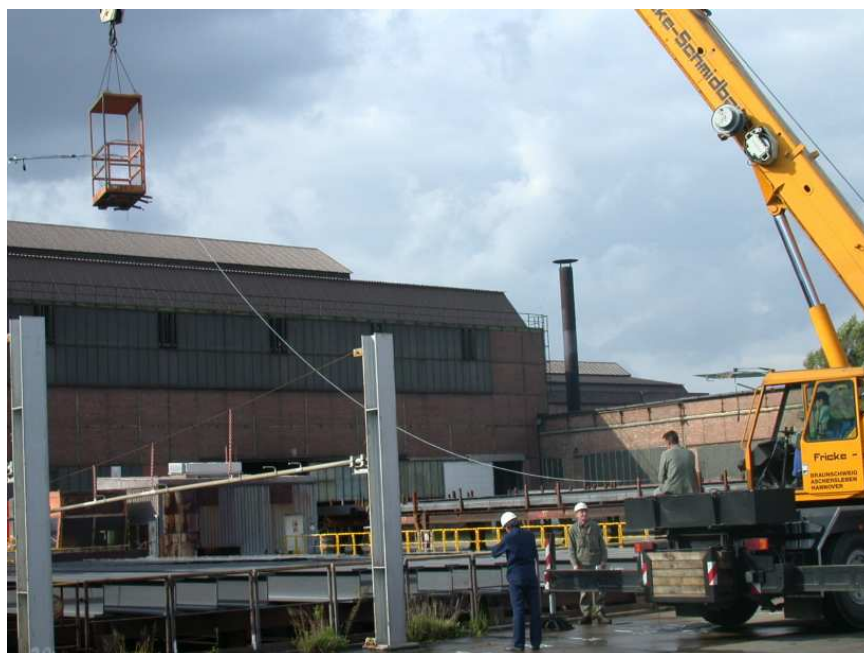
Figure 21. Crane with measurement equipment during the first path. Picture courtesy of PTG.
